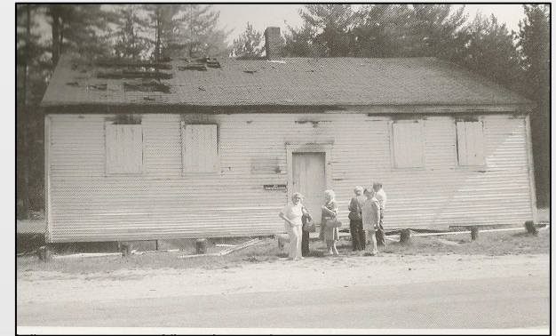
THE DAMAGE AFTER THE JULY 1985 FIRE.
